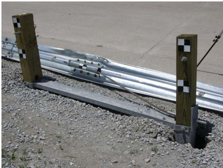
Figure 63. System Anchor Damage, Test No. LSC-2
