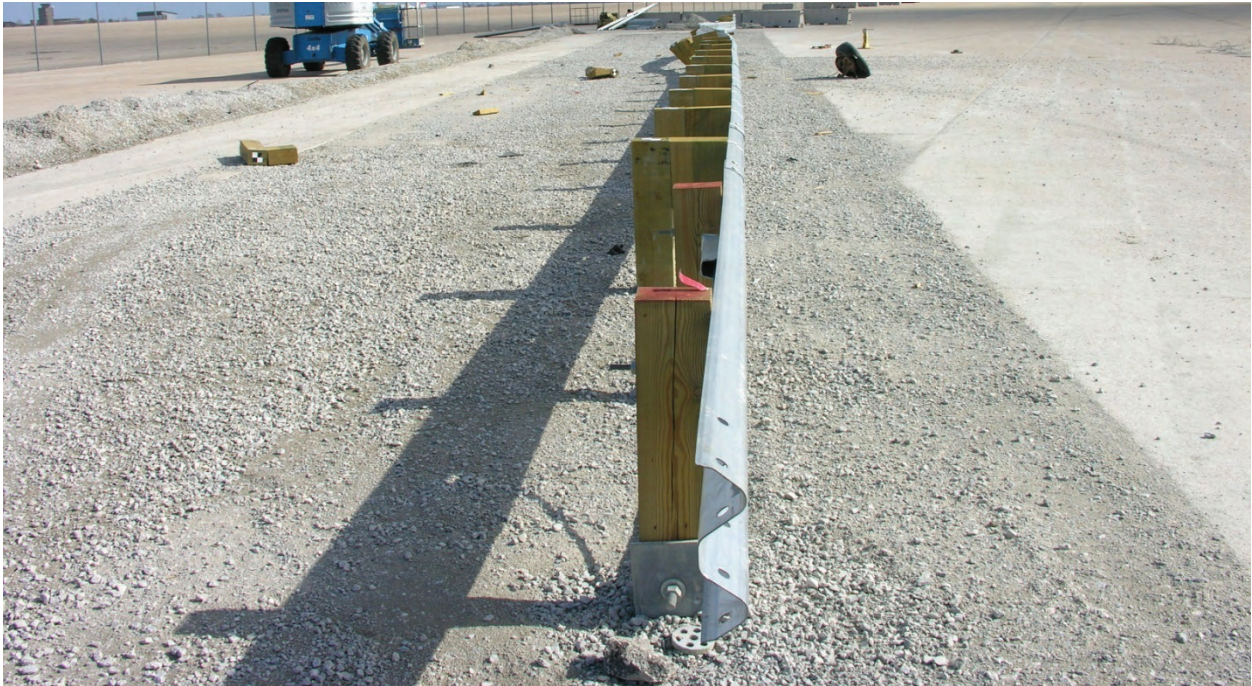
Figure 29. System Damage, Test No. MGSWP-1
