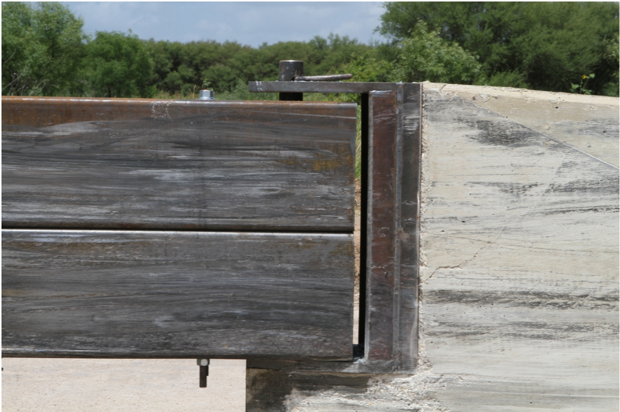
Figure 6.4. TxDOT Median Barrier Gate after Test No. 420020-6.
