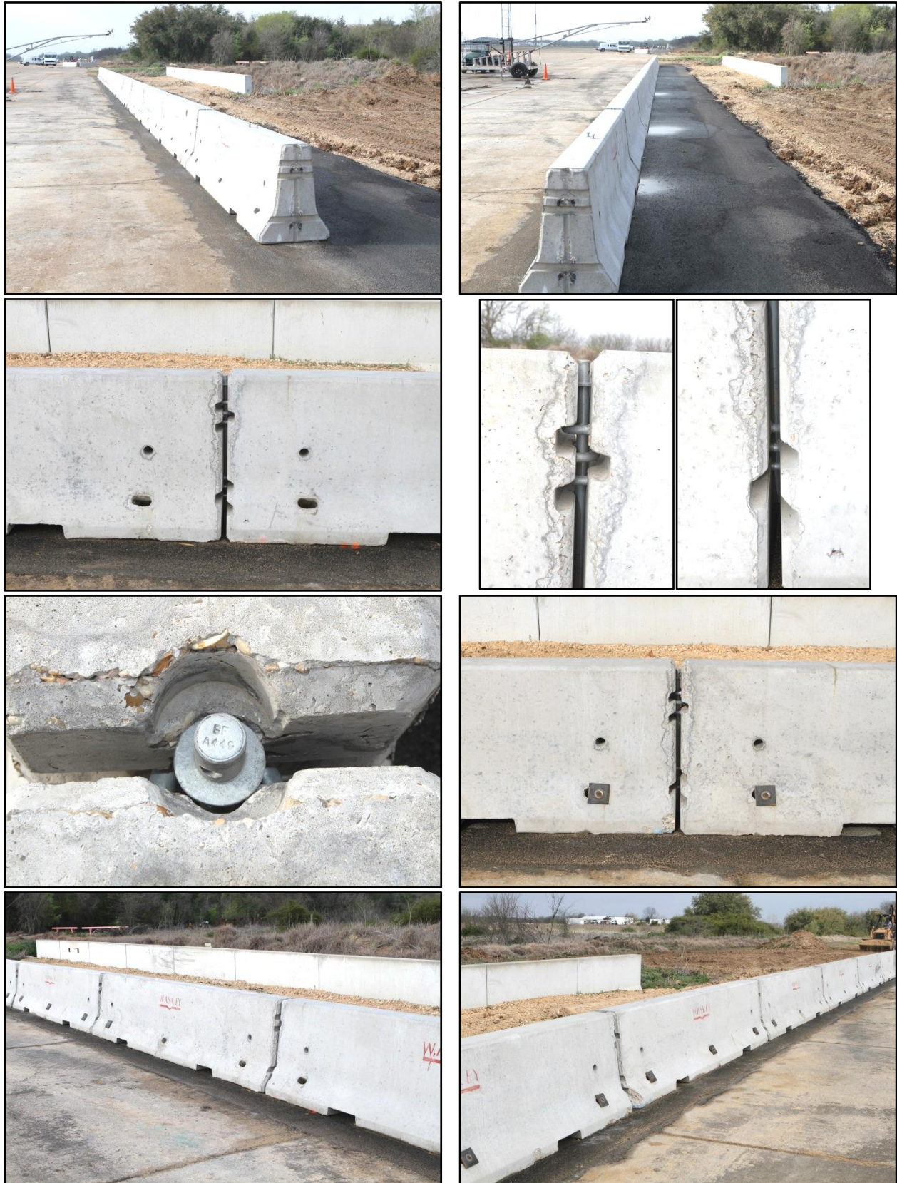
Figure 5.6. Transition from free-standing F-shape barrier to pinned F shape barrier on asphalt prior to test 601651-1.
