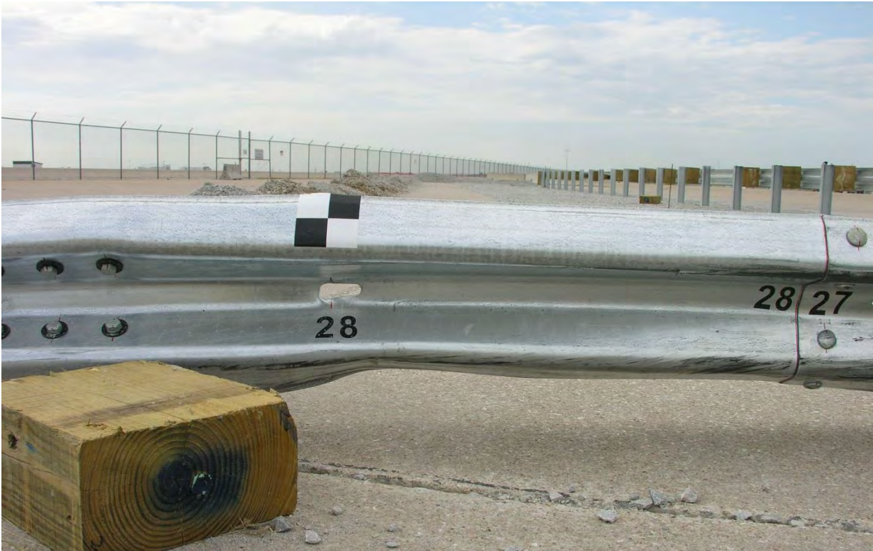
Figure 137. Rail Slot Tearing at Post Nos. 24 and 28, Test No. WIDA-1
