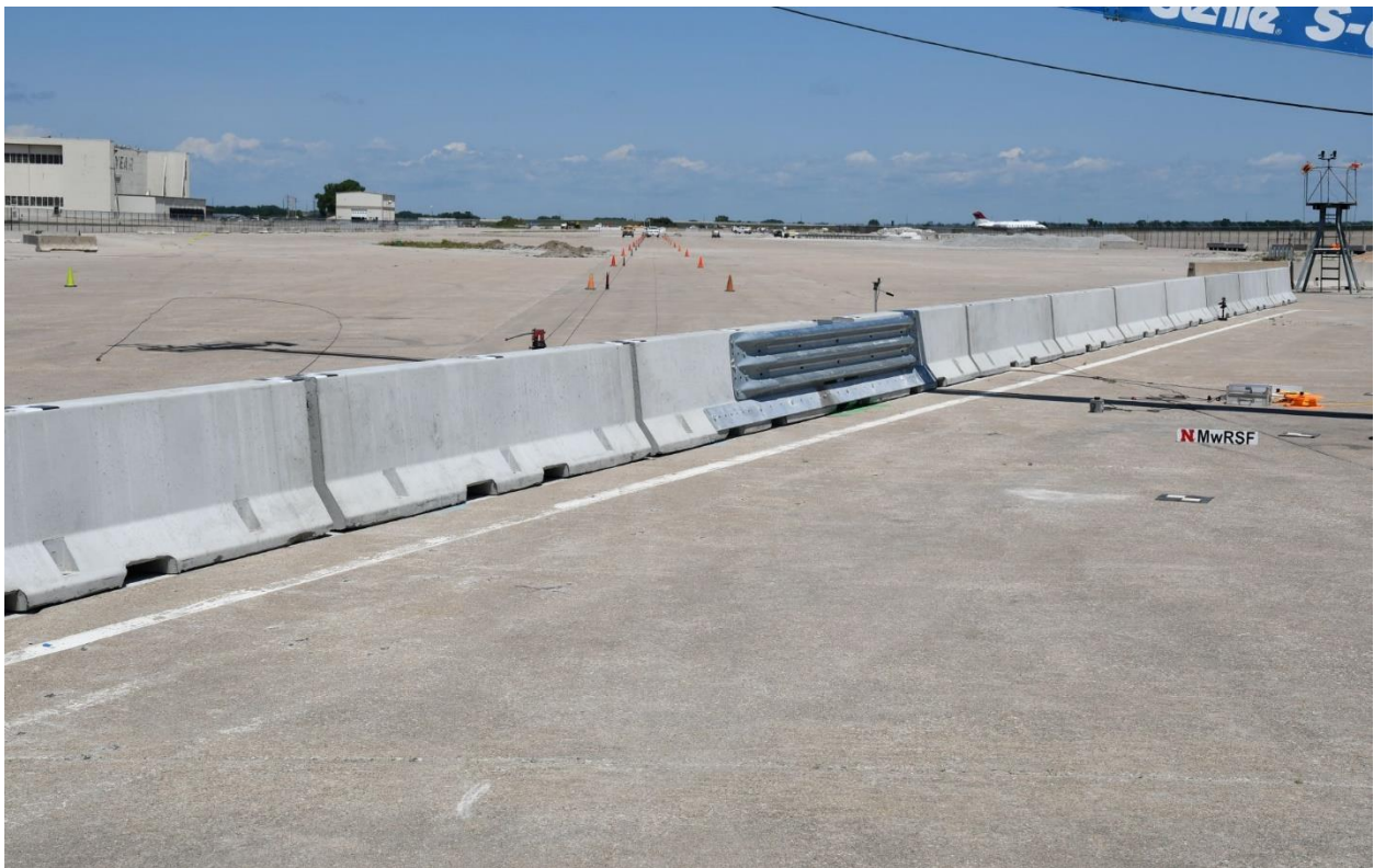
Figure 62. Test Installation Photographs, Test No. GSH-2
