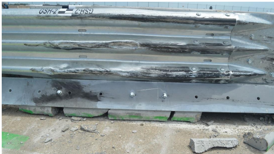
Figure 74. Thrie-Beam and Barrier No. 9 Damage, Test No. GSH-2
