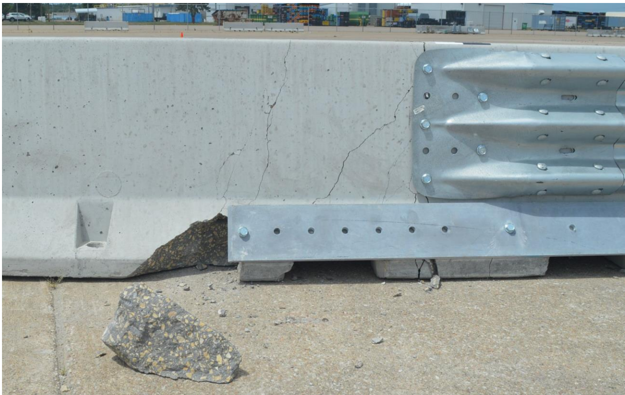
Figure 75. Barrier No. 9 Damage, Test No. GSH-2
