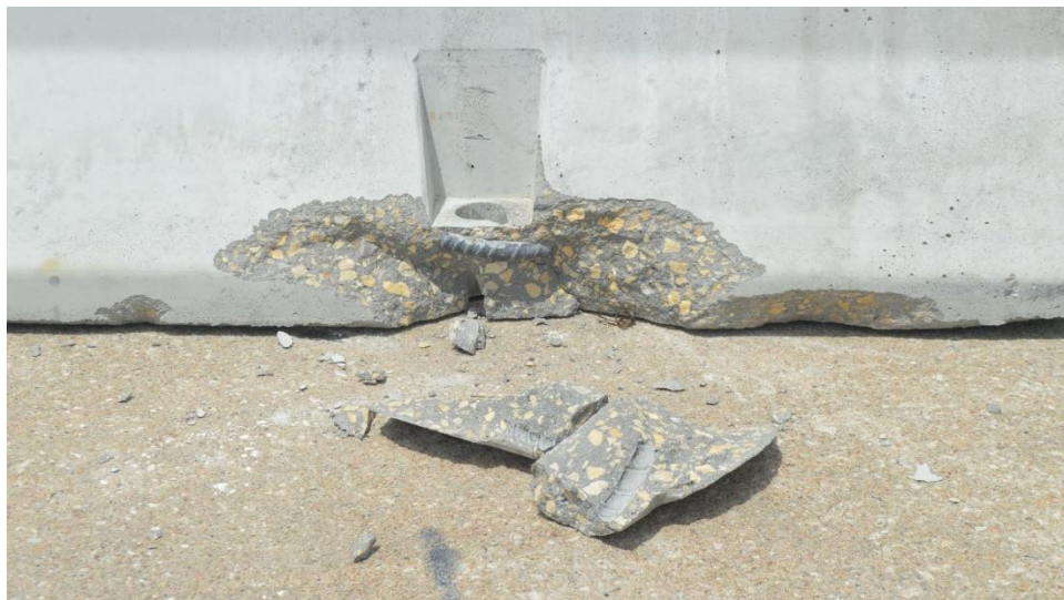
Figure 78. Barrier No. 11 Damage, Test No. GSH-2
