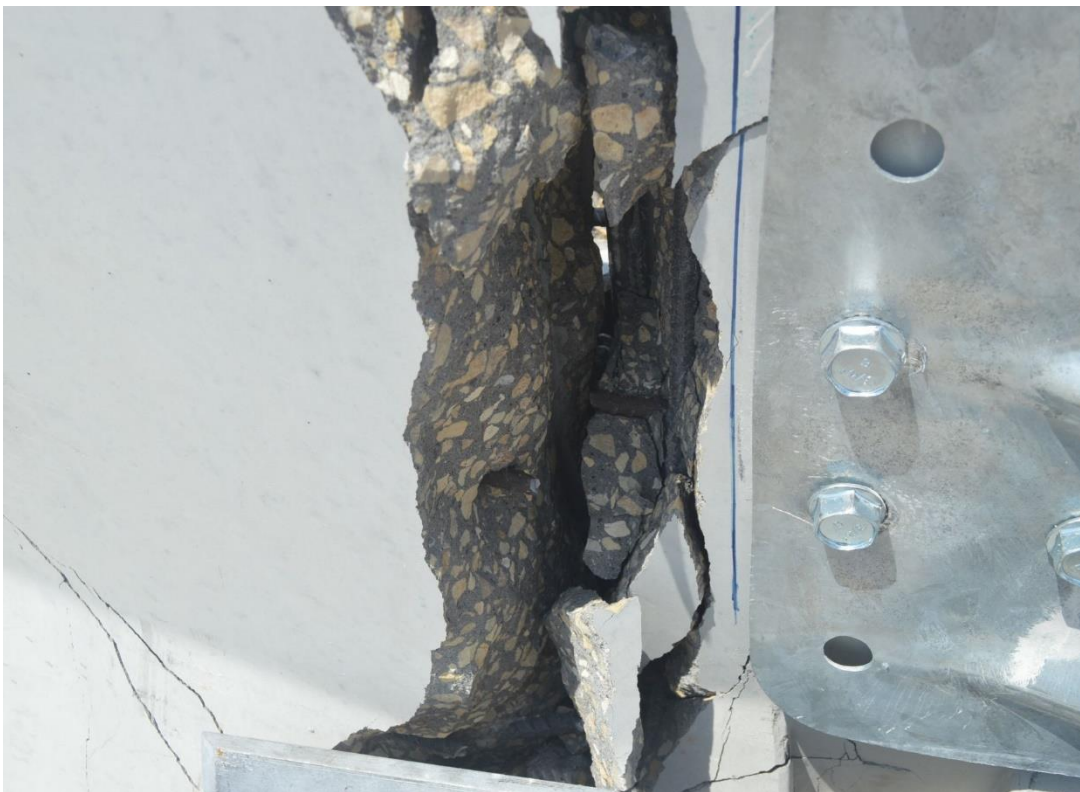
Figure 40. Longitudinal Rebar Shear, Non-Traffic Side, Barrier No. 9, Test No. GSH-1
