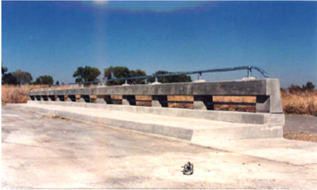
Figure 2-3 View of the Completed Barrier Type 80SW and Sidewalk System (Meline et. al, 1999)
