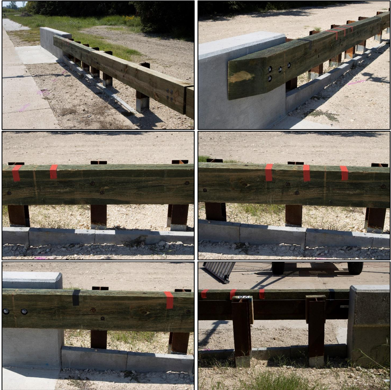
Figure 6.2. Merritt Parkway Guiderail Transition prior to Testing.
