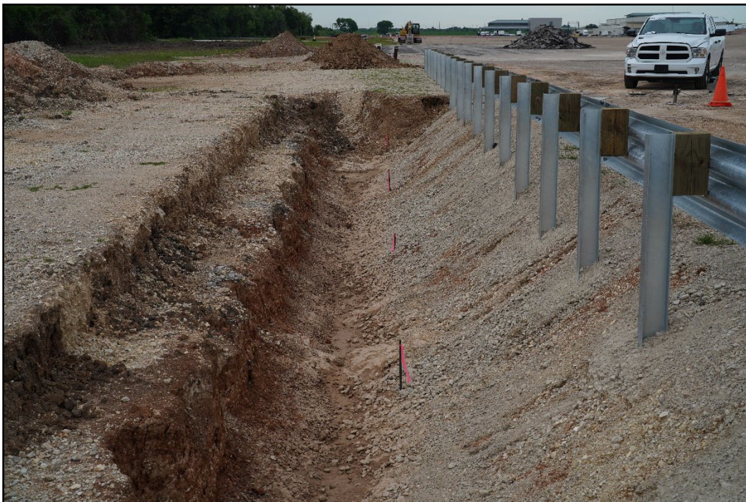
Figure 3.5. Field Side View of the Guardrail System on 1:1 Slope Prior to Testing.
