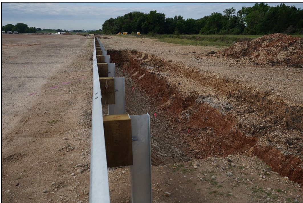
Figure 3.3. Upstream In-Line View of the Guardrail System on 1:1 Slope Prior to Testing.
