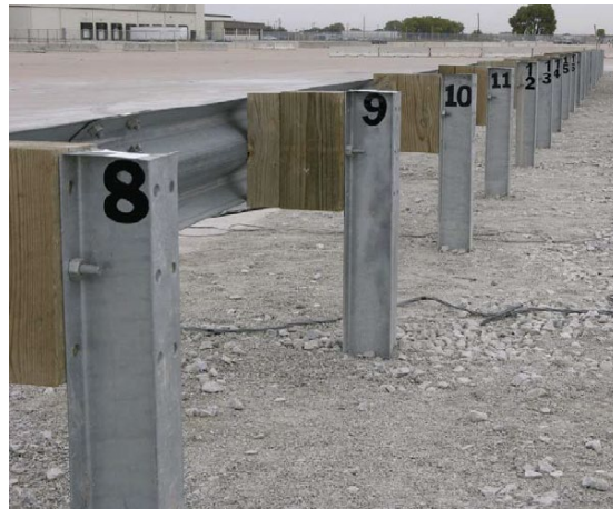
(b) Installation Before Test
