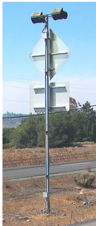
Figure 1.1. Sign Support System with Flashing Beacon Equipment.
