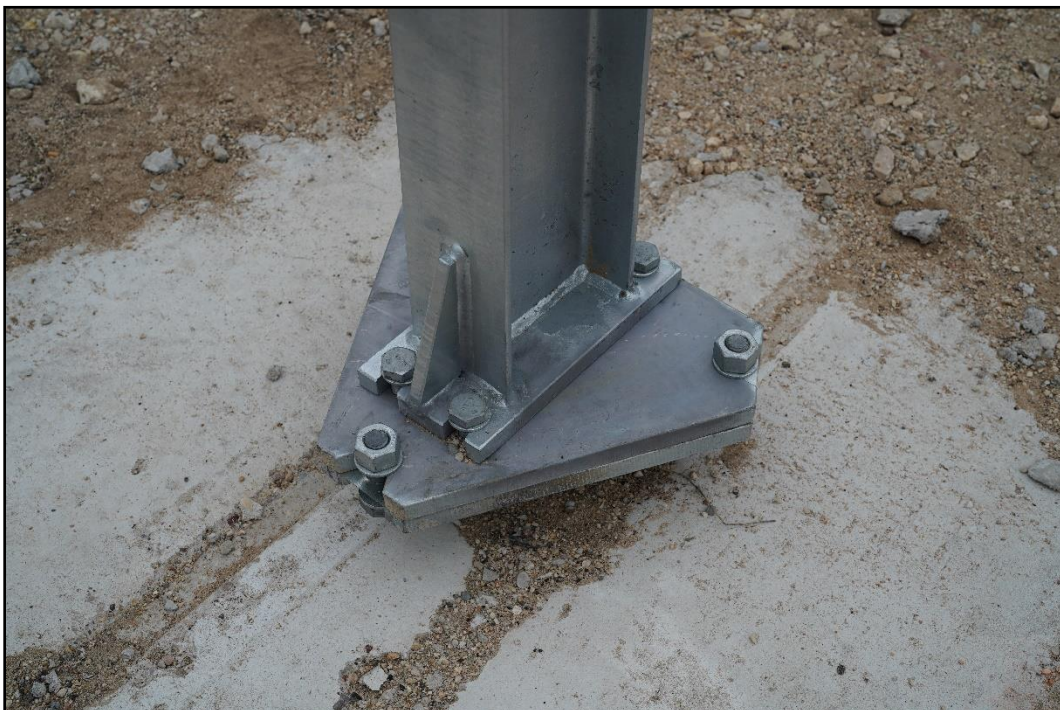
Figure 4-12. Slip Base on the Guide Sign with Large Sign Supports prior to Test 616401-01-3.
