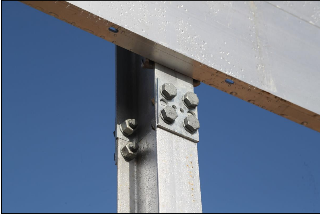
Figure 4-26. Fuse plate on the Guide Sign with Large Sign Supports prior to Test 616401-01-8.
