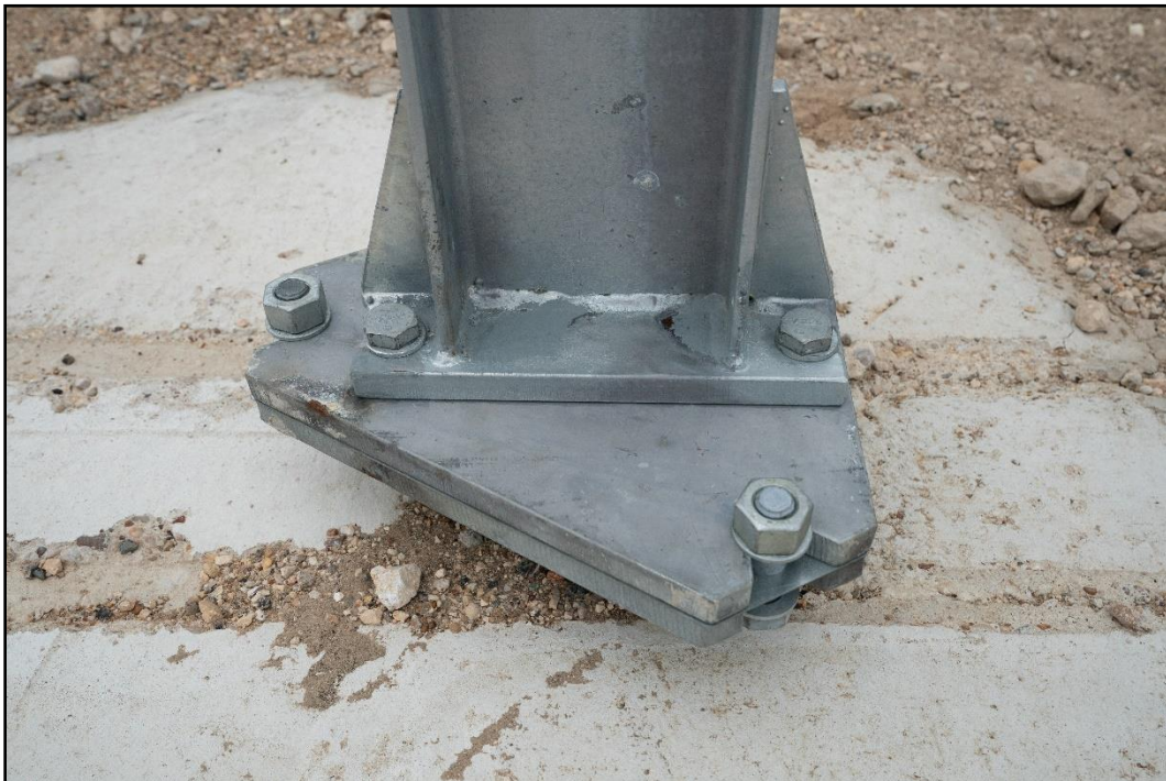
Figure 4-17. Slip Base on the Guide Sign with Large Sign Supports prior to Test 616401-01-9.
