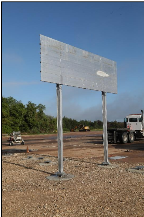
Figure 4-24. Impact Side of the Guide Sign with Large Sign Supports prior to Test 616401-01-8.
