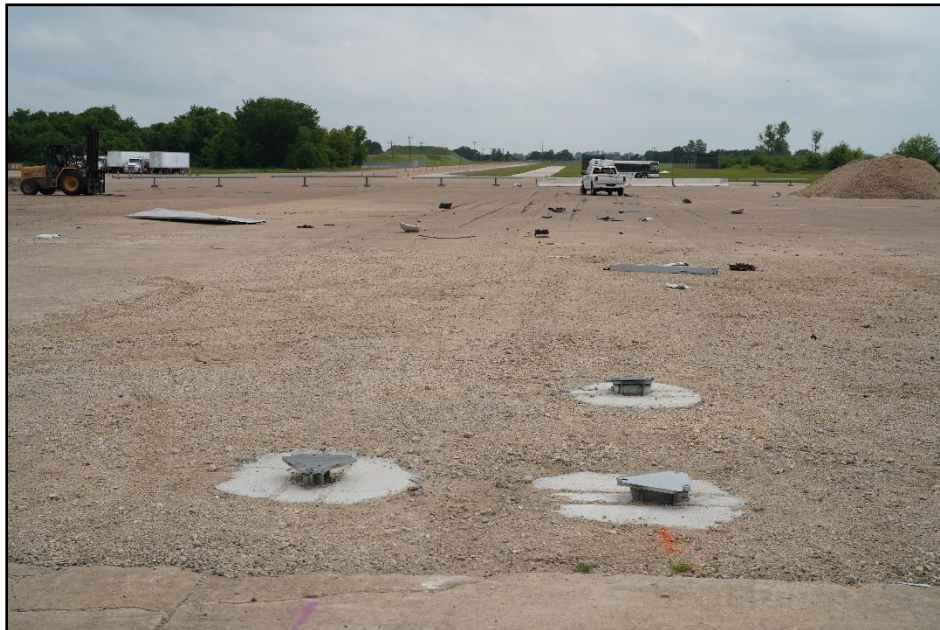
Figure 9-5. Guide Sign with Large Sign Supports at Impact Location after Test 616401-01-3.
