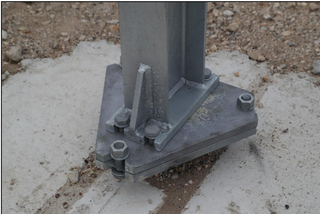
Figure 4-22. Slip Base on the Guide Sign with Large Sign Supports prior to Test 616401-01-4.
