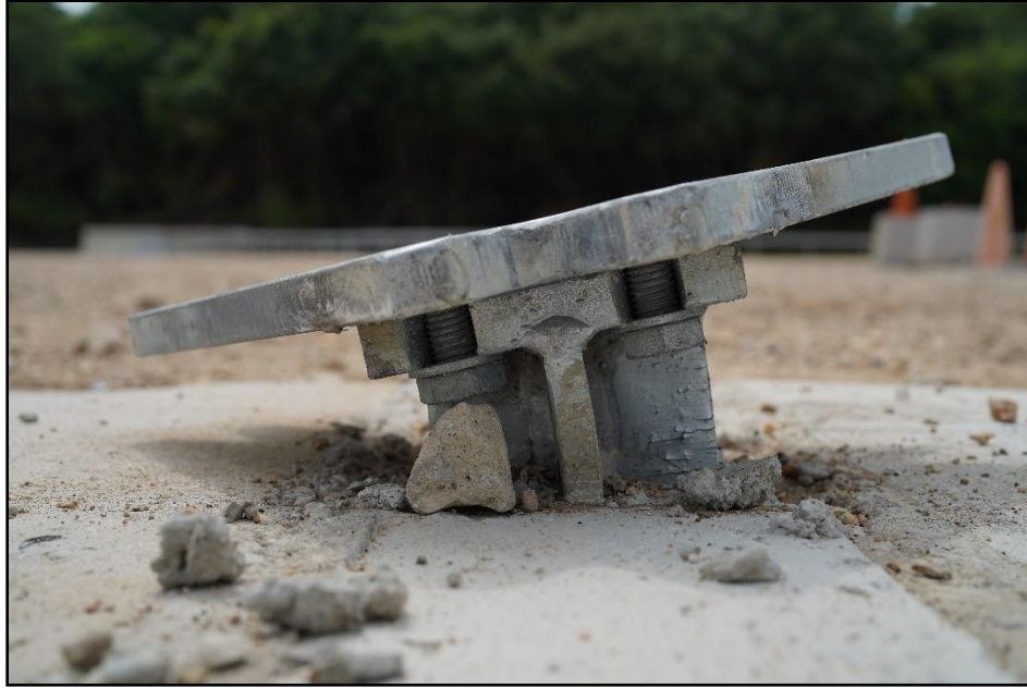
Figure 9-6. Footer for the Guide Sign with Large Sign Supports after Test 616401-01-3.
