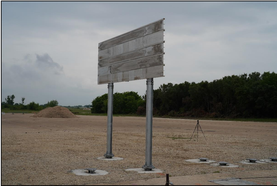
Figure 4-9. Impact Side of the Guide Sign with Large Sign Supports prior to Test 616401-01-3.
